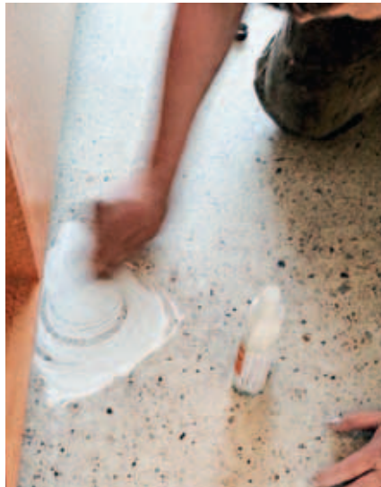
Even an oiled concrete floor can be repaired. Here using a wet-on-wet method, the surface is being repaired after leaking battery acid affected the surface sheen.
