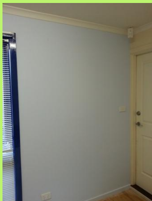
6. Next day, no sign of the repair and no roller marks.....yeh.
